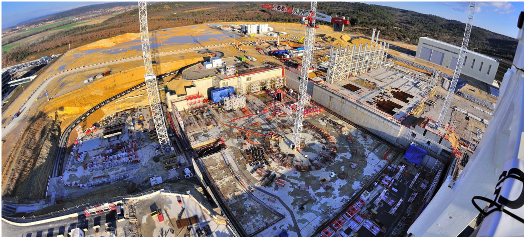
Status of the ITER construction site as at February 2015 (photo: ITER Organization)
